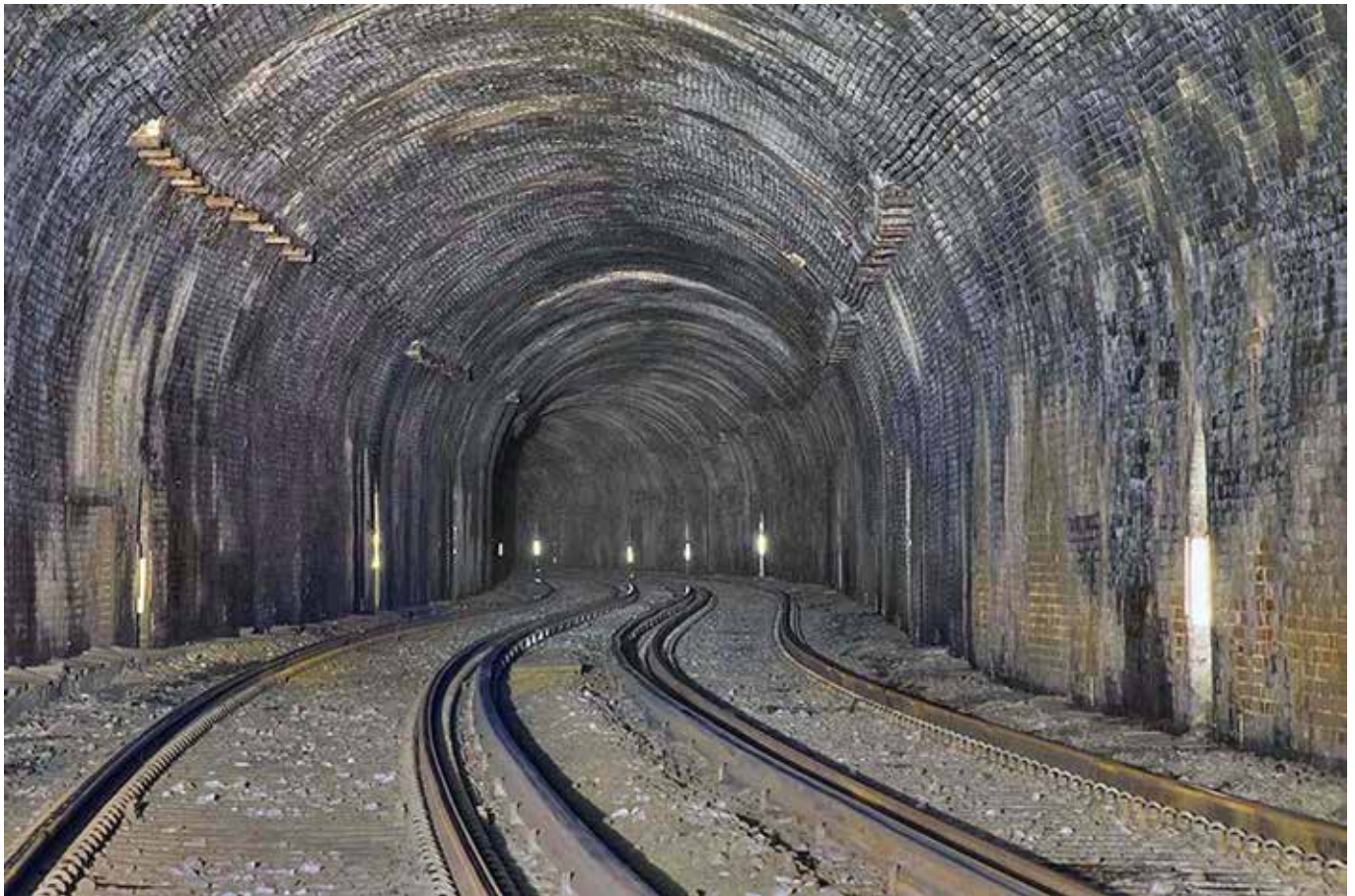
Interior of tunnel showing the double curvature. The radius of the curves is probably exaggerated in the photograph
